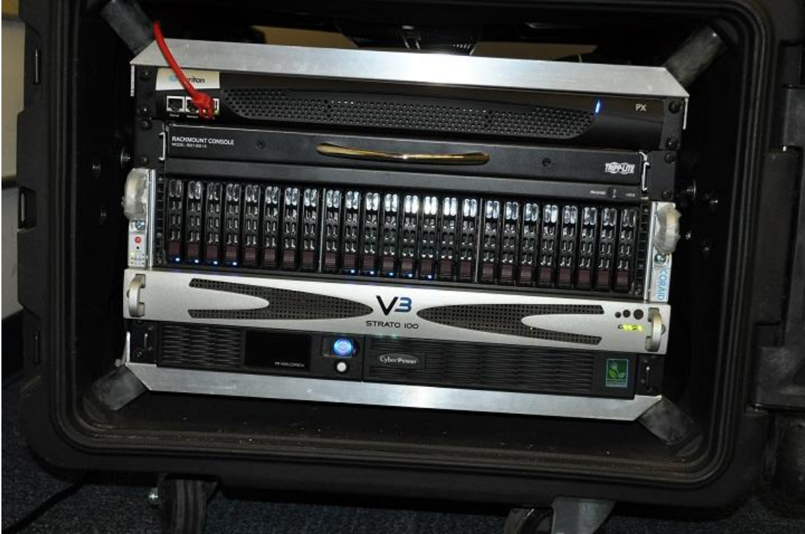
Figure 7. EOC in a box showing from top to bottom: Raritan PDU, TrippLite KVM, CORAID SAN, V3 Server, and CyberPower UPS.
