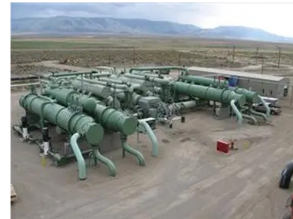
~36MW Binary-Cycle Geothermal Electrical Generating Plant in Raft River, Idaho
